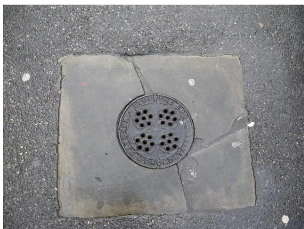
Cast iron coal hole cover in Edgar Road
